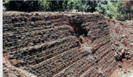
The reinforced rockfall barrier after the impact shows minimal damage.
