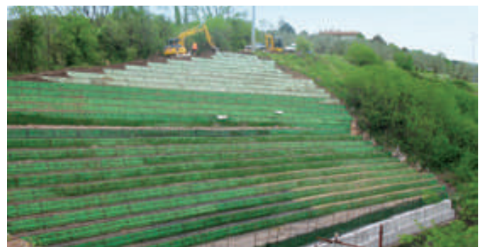
Repair of a collapsed slope in Serravalle Pistoiese on the Firenze-Lucca railway line.
