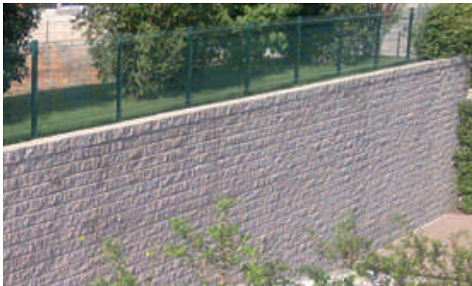
Connection with fence.
