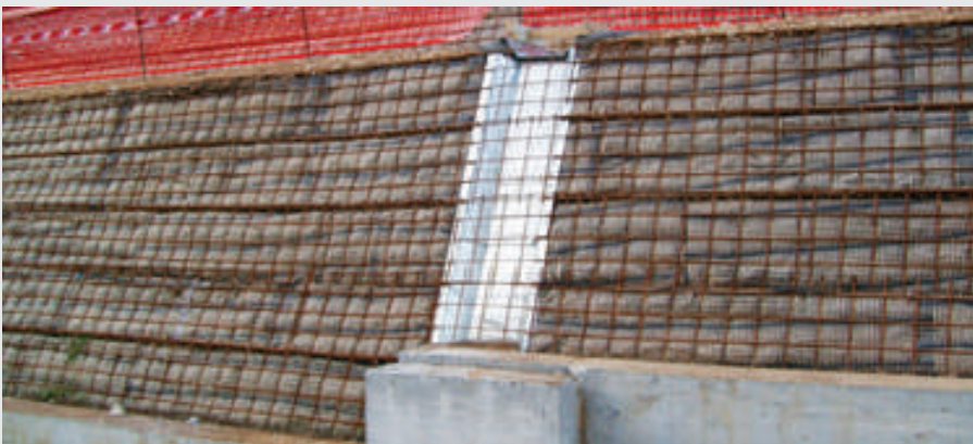
Creation of bends and corners. Positioning of metal roof tiles for the outflow of surface water.
