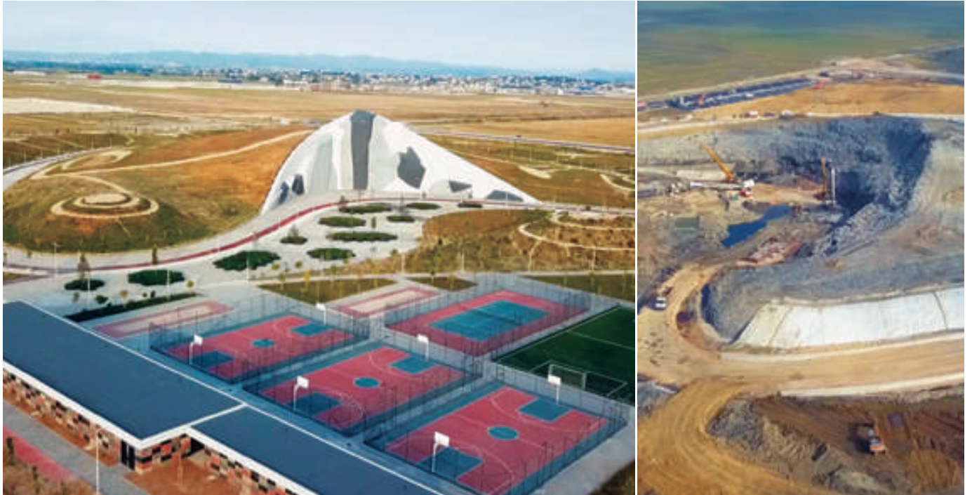
Ecopark Durazzo: 21 m high reinforced embankment to reduce thrust on a 28 m high concrete climbing wall.
