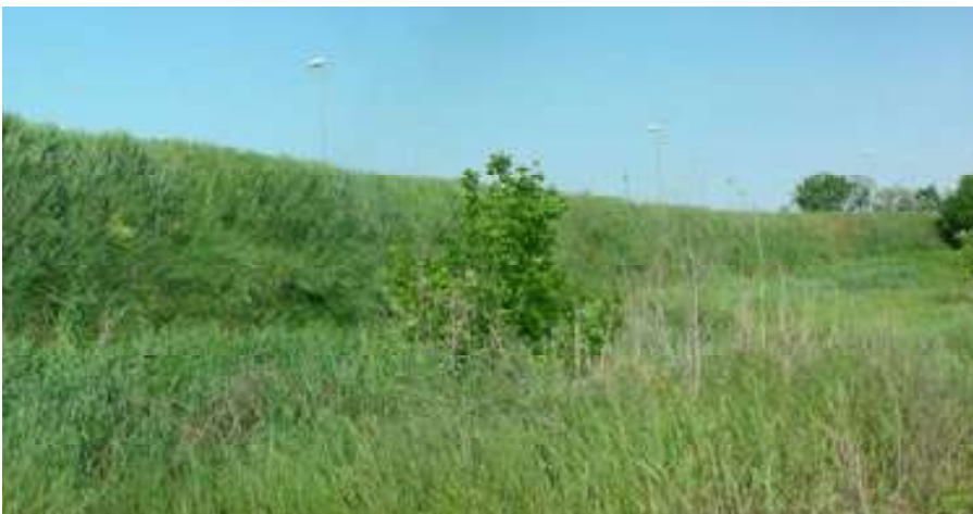
Northern Ring Road of Pavia. Construction of a 400-meters-long noise barrier and wing walls using vegetated reinforced slopes, covering a total face area of 2500 square meters.
