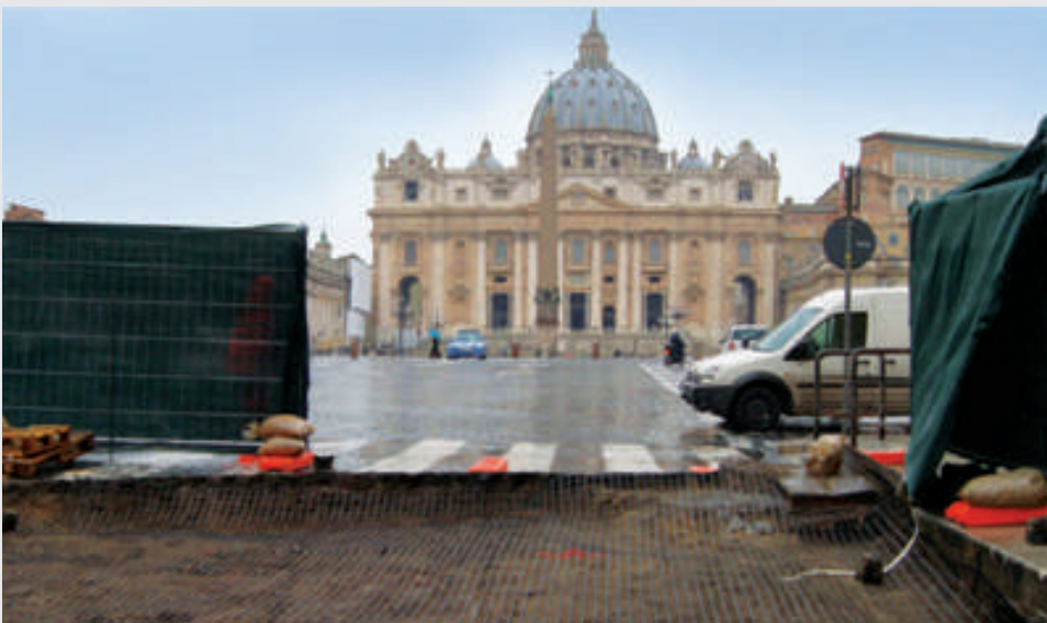
Rome, St. Peter's Basilica. Stabilization of the floor adjacent to the basilica using the TENAX 3D GRID XL product.
