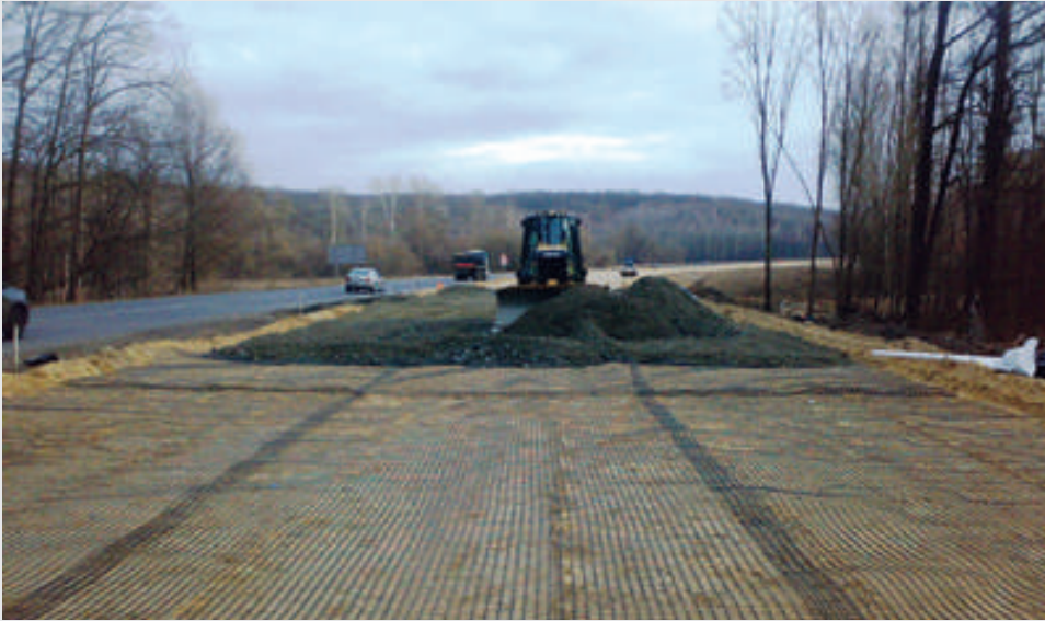
Ukraine, application of TENAX 3D GRID XL geogrid to stabilize a road.
