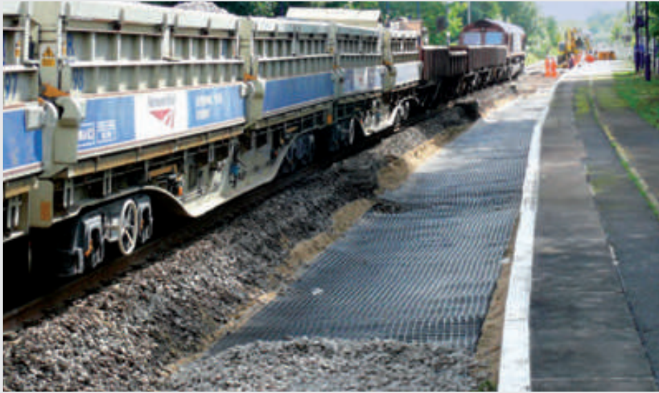
Midgham, England. TENAX geogrids installed to increase ballast performance and reduce maintenance frequencies.
