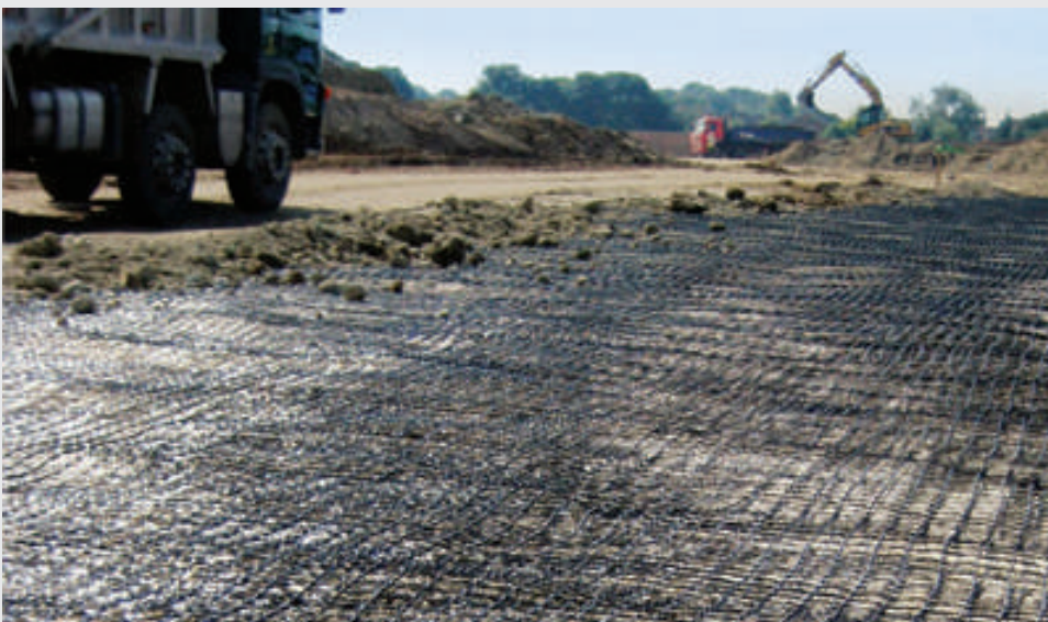
Abraham Darby Academy, Telford, Shropshire. Application of 10,000 m 2 of TENAX 3D GRID MS geogrid for soil stabilization before the construction of a primary school.
