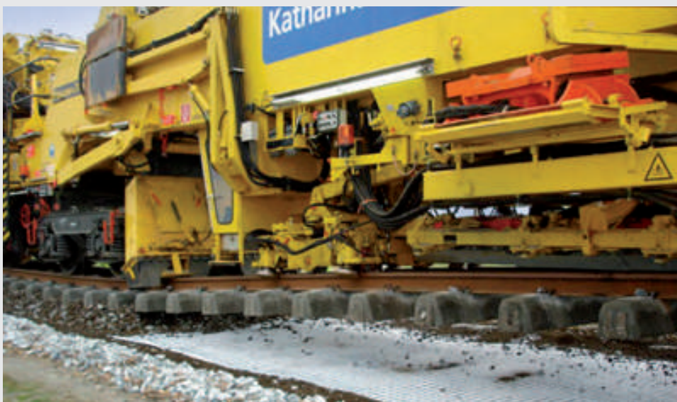
Mantgum, Netherlands. The ballast refurbishment of the Frisian track was completed using a ballast cleaning train traveling at 3 m/s whilst simultaneously placing a geocomposite to stabilize the ballast/subgrade interface and to minimize the upward movement of the background.
